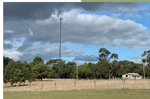
A mobile tower providing a network
